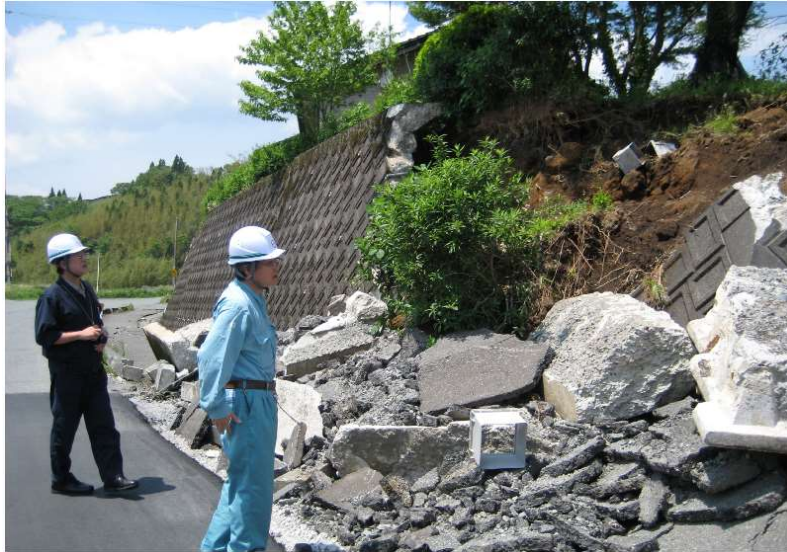
(a)練積み擁壁崩壊
